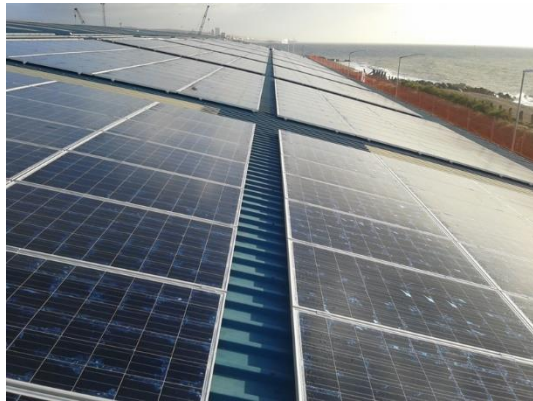
Solar panels on warehouse roofs
